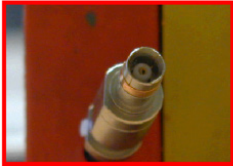
Figure 4-6 Incorrect connector (fixed)
